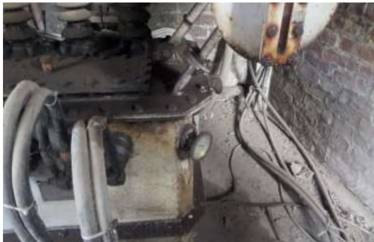
Figure 6. Snapshot taken during factory visit (Oil leaking in an old transformer)
