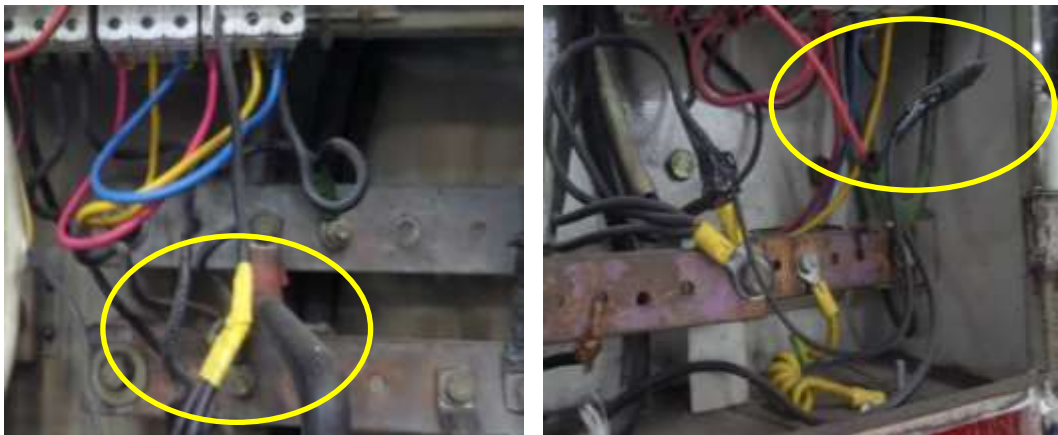
Figure 4. Snapshot taken during factory visit (PVC tape wrapping to insulate twisting joint)
